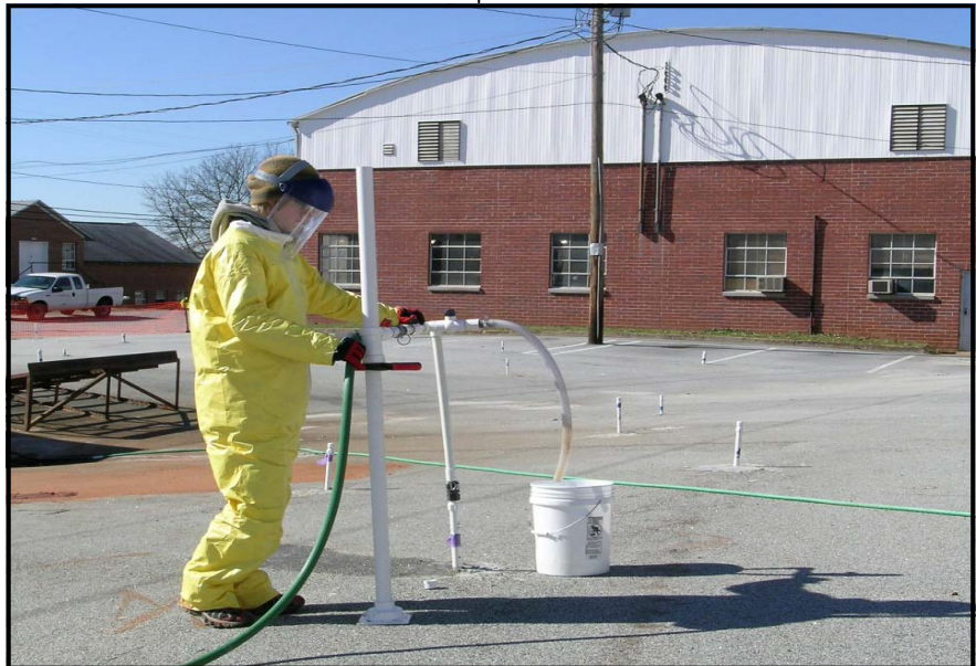
Project cleanup at the Griffin Campus around the future Student Learning Center.
