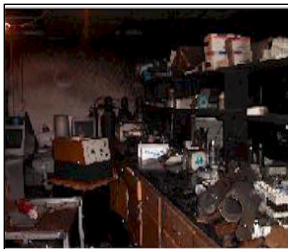
Another part of the room and the damage caused by extinguishing the fire and securing the room from further fire outbreaks.
